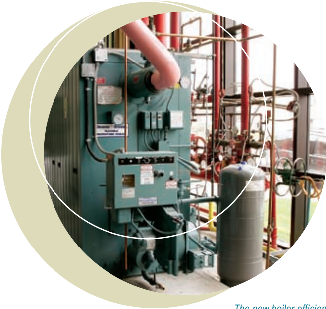
The new boiler efficiently heats water to 200 degrees Fahrenheit.
